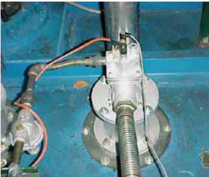
Kromschroder flame-management system, combined with other upgrades, reduced furnace fuel consumption by 40%.
