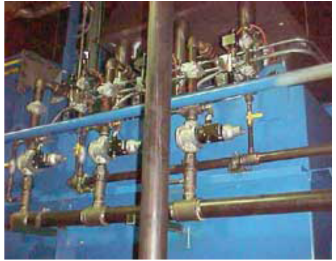
Six Kromschroder BICR single-ended, self-recuperating burners, a flame-management system, and Kanthal APM radiant tubes reduced gross heat input to the furnace by 22%.
